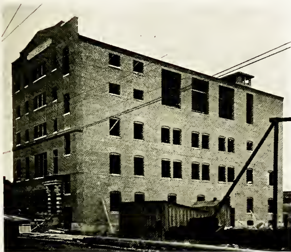
The J. B. Carr Biscuit Co. Factory Building North Pennsylvania Ave. (Under Construction)
